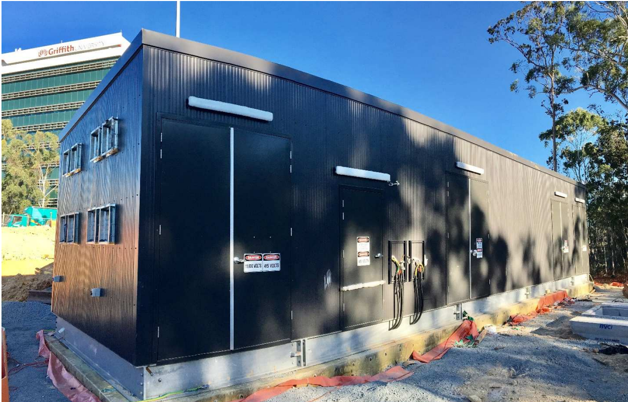
Traction Power Substations (TPS) located at the corner of Olsen Avenue and Wintergreen Drive, Parkwood.
