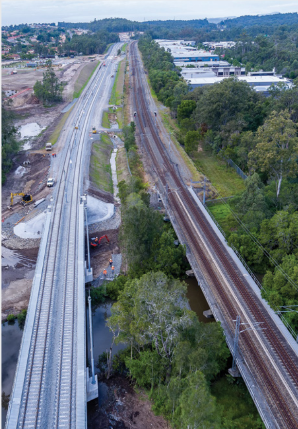
LIGHT RAIL TRACK AT COOMBABAH CREEK READY FOR TESTING AND COMMISSIONING.
